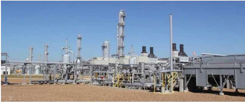
FIGURE 2: A view of Kinder Morgan’s Houston Central Plant, which processes NGLs.
